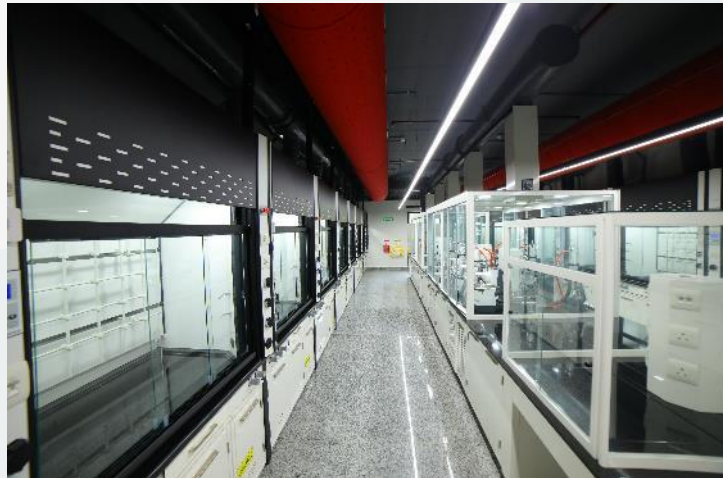
Discovery Expansion at R&T Centre, Hyderabad
